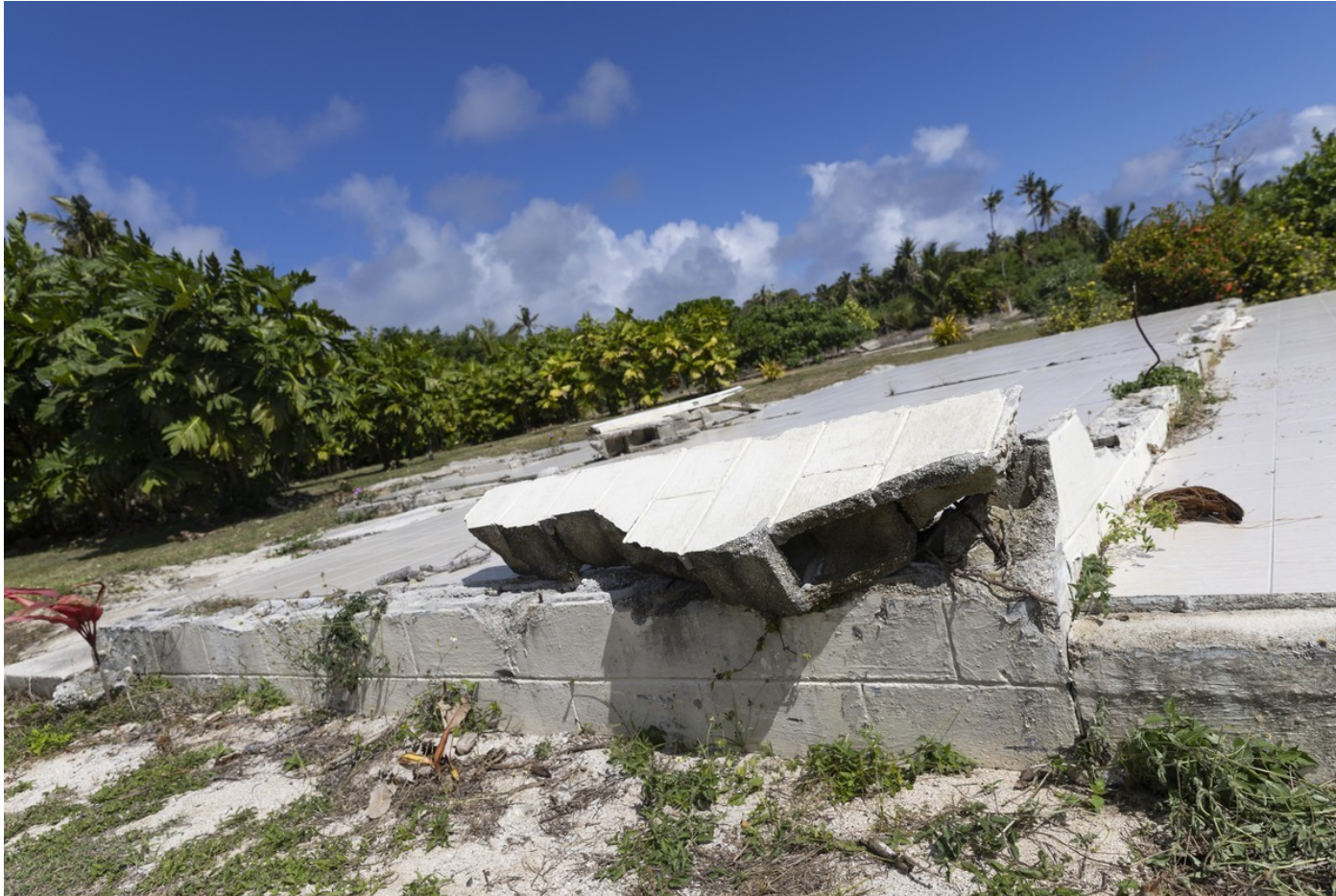
A damaged sea wall in Tonga/Kiara Worth
