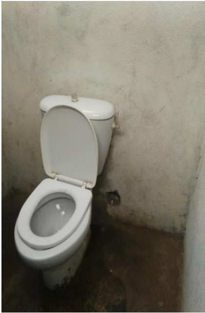
Toilet without piping...
