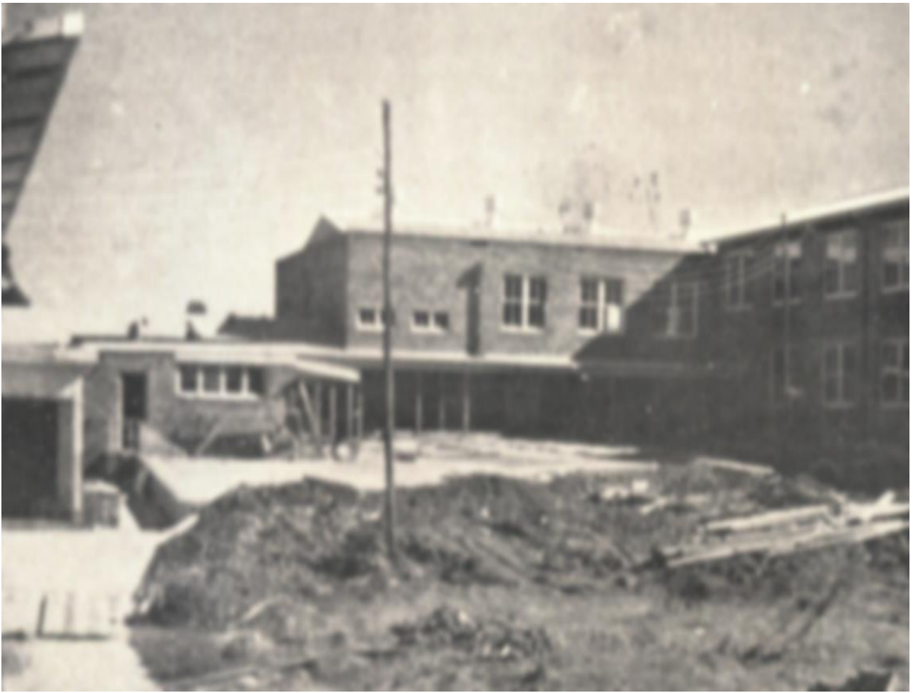
Construction of Penrith High School. Our Club has made significant contributions to the school over the past 70 years.
